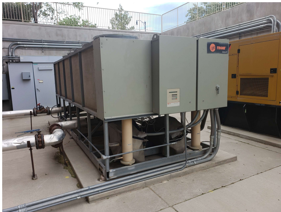
Photo: New chiller unit at city hall
